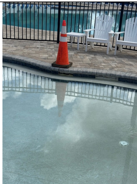
Photo 3: Damaged Coping and Waterline Tile
