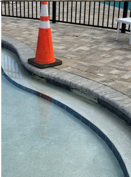
Photo 2: Damaged Coping and Waterline Tile
