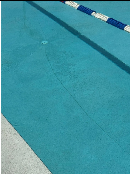
Photo 8: Lap Pool Floor Cracks
