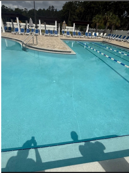
Photo 5: Crack Between Main Pool and Lap Pool
