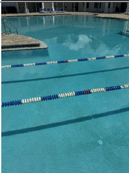
Photo 6: Lap Pool Floor Cracks
